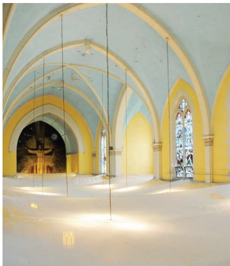
The roof and ceiling at St. Francis of Assisi Church, Toronto will be repaired.
