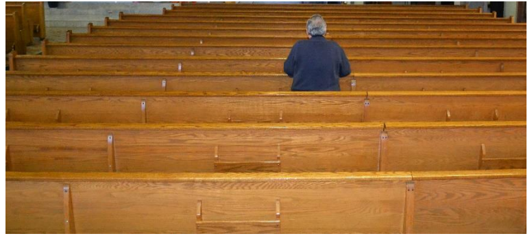
At St. Philip Neri Church, the solid oak pews have become worn over time. The parish will refinish the pews to provide a comfortable environment in which all parishioners can worship.
