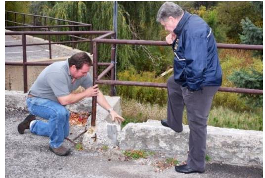
At St. David's in Maple, the parish will use its share of campaign proceeds to undertake important major repairs including this cracked and crumbling retaining wall.
