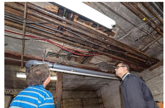
St. Clare’s Church in Toronto is an historic and beautiful building. The parish will devote part of its share of the Family of Faith campaign toward repairing its heating, cooling, electrical and lighting systems.
