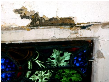
St. Brigid's church requires capital repairs which will be addressed as funds become available.
